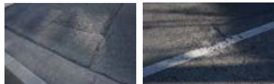
Figure 3: Example of potholes and cracks.
