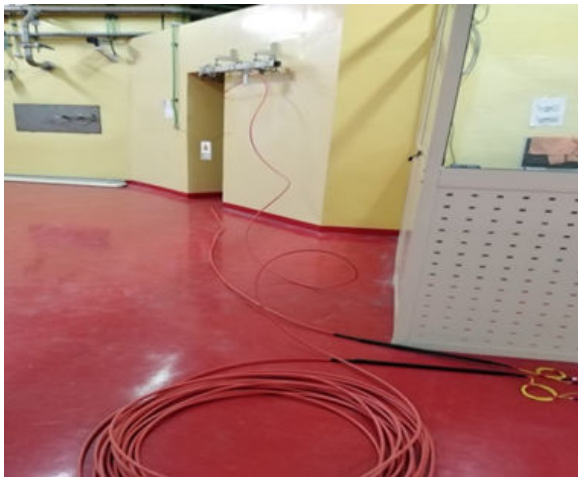
Figure 3: Telecom Egypt fiber cable within spliced connectors.
