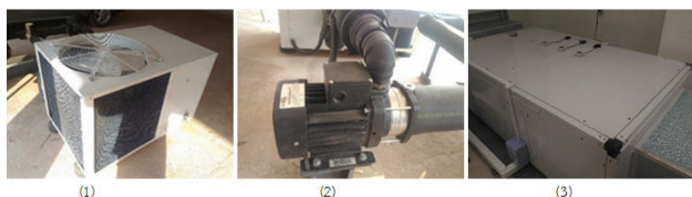
Figure 10: A Chilled water for air conditioning system (1) Air-cooled chiller, (2) Chilled Water Pump and (3) Air Handling Unit.
