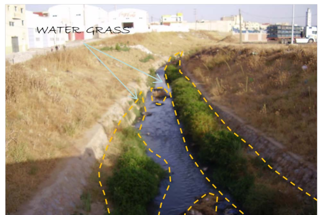
Figure 11: Water grass on the floor and edge of the channel.
