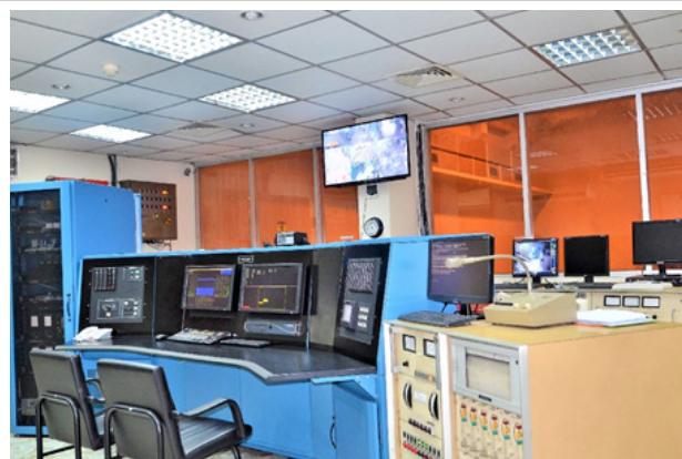
Figure 1: BTRR control room.
