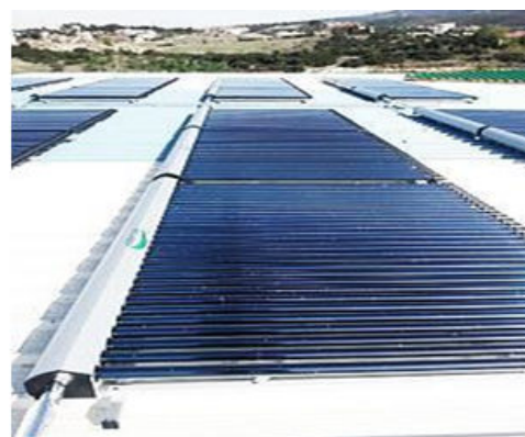
Figure 1: The evacuated tube solar fins. It is made up of a series of parallel clear glass tubes connected to a header pipe that replace the darkened heat absorption panel.
