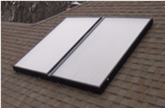
Figure 2: The solar collector with a flat plate. It's a metallic box with a top cover made of plastic or glass and a dark-colored absorber plate on the bottom.
