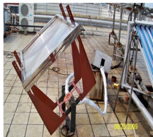
Figure 4: Illumination system using fibre optics and PV system.
